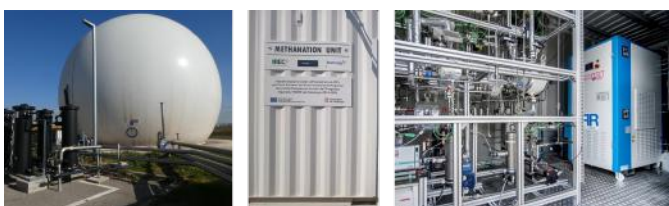
Methanation unit in EDAR (Sabadell)
