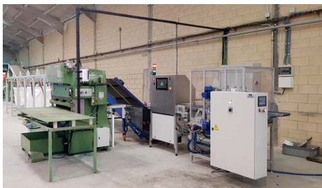
Sorting system - Pilot line for recycling plastic in Lurederra (Navarra)
