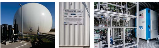
Methanation unit in EDAR (Sabadell)
