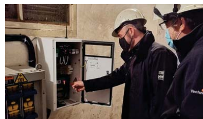
Cyber-attack feature validated in Estabanell grid
