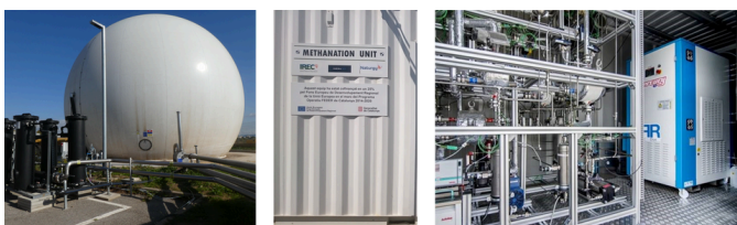
Methanation unit in EDAR (Sabadell)
