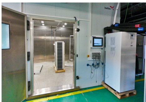
Heat pump in our testing lab
